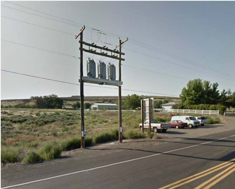
Voltage Regulator SCADA Automation
