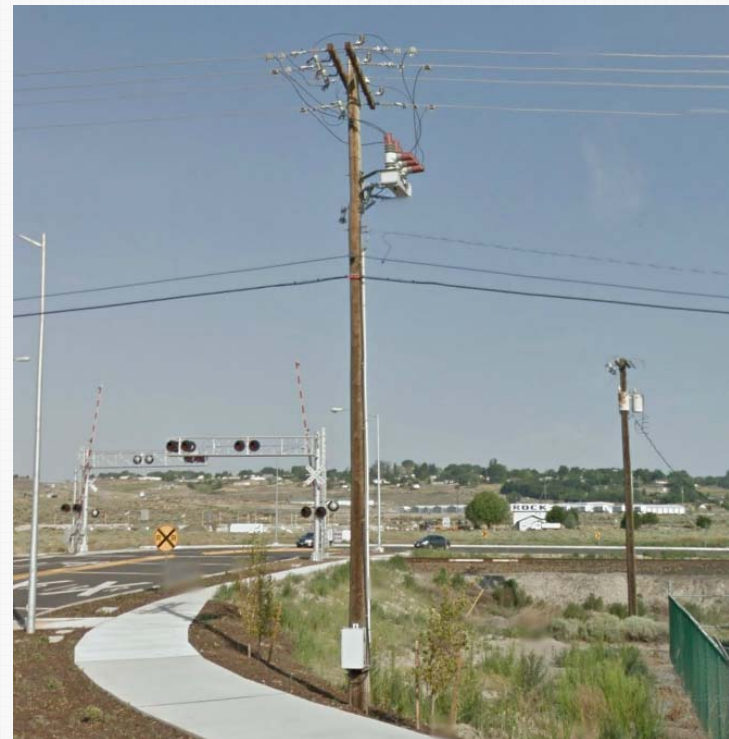
Recloser (Circuit Breaker) SCADA Automation
