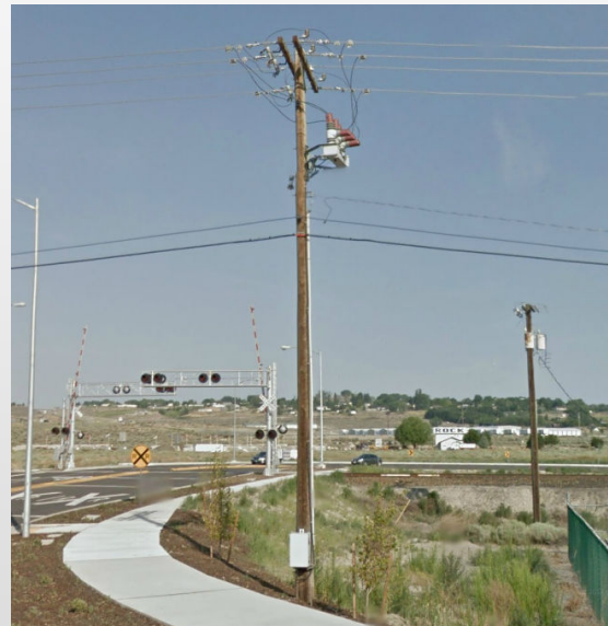
Reclosers (Circuit Breakers)
