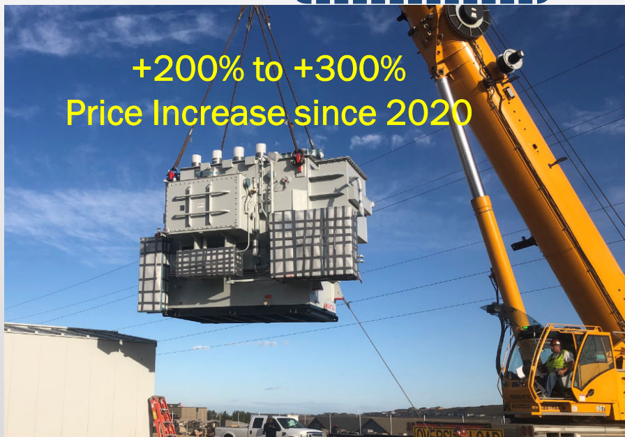
25-megawatt Substation Transformer
